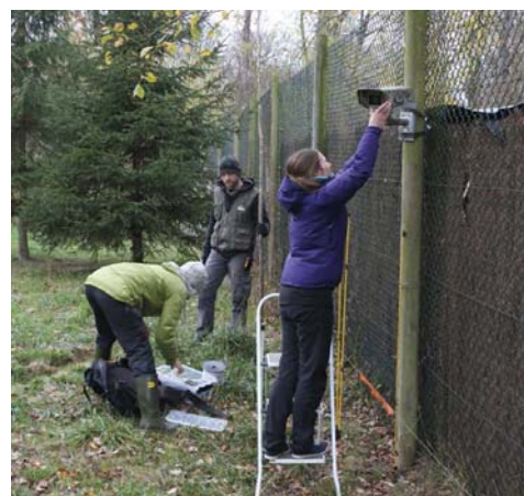
Fig. 2. Installation of the camera equipment: remote camera (Bushnell, above) and thermal camera (AXIS Q1921-E, below).
